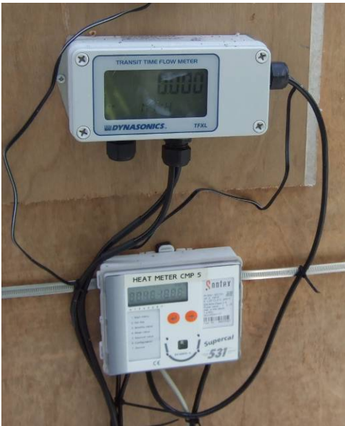
Figure 8. Heat meter for block 5
